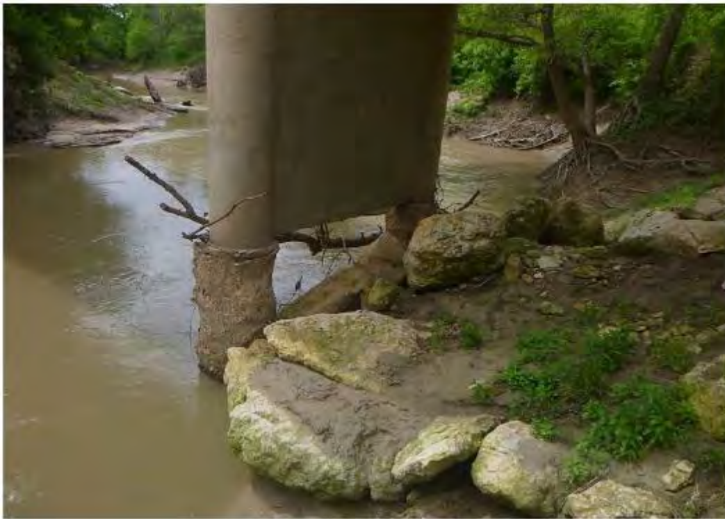
Figure 47. Local scour erosion with 10.5 feet of bridge pier exposed, 2020. Photo by TxDOT.
